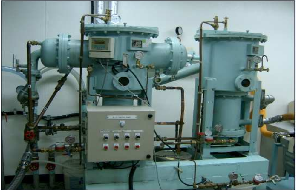
Photo.3.1 2 stage fresh water generator
