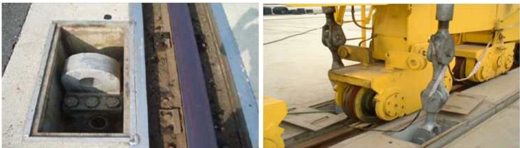
Fig. 2.12 Tie down of the port crane(2)
