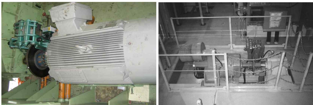
Fig. 2.7 Trolley traversing unit of the STS crane
