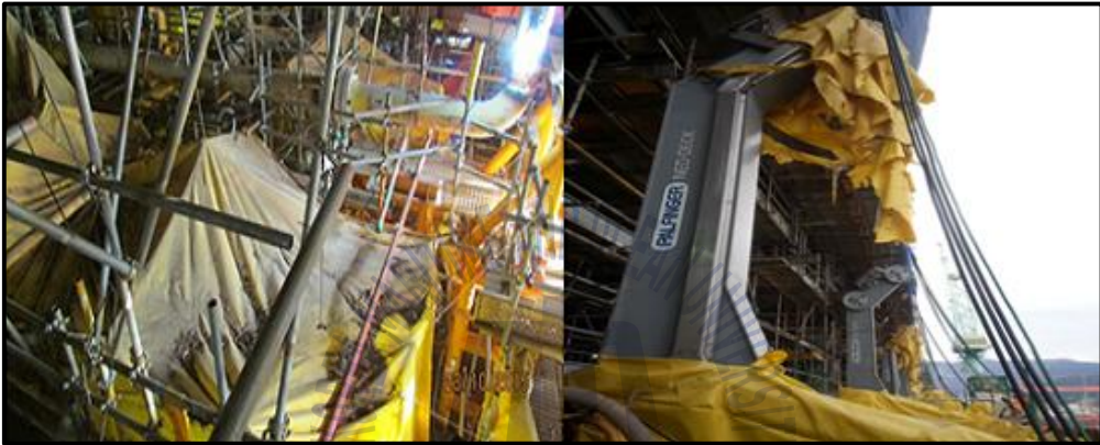
Fig. 4.11 Protection cover damage
