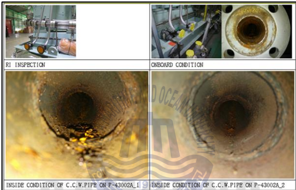
Fig. 4.12 Flange protection cover missing
