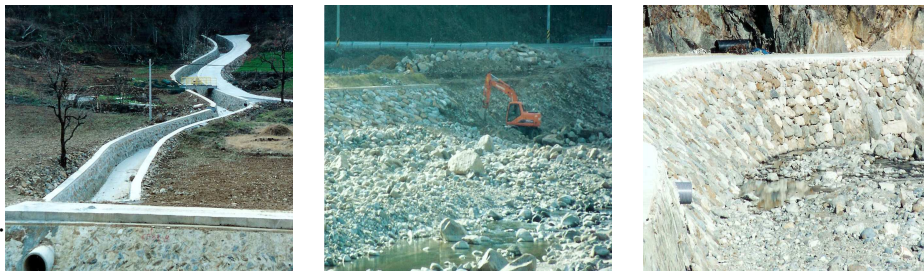
Fig 1.1 Restoration the present position of damage by a flood
