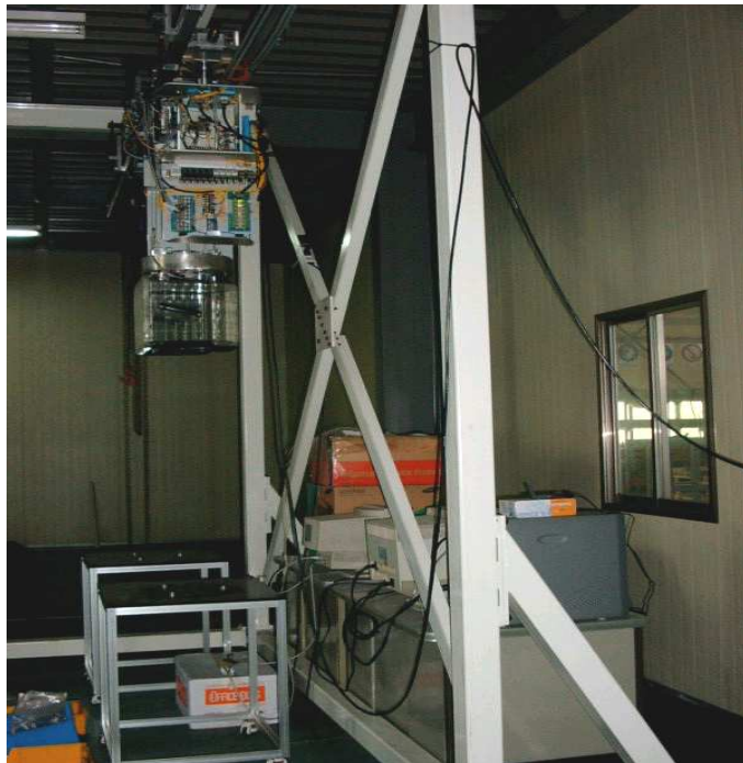
Fig. 5.19 OHT Hoist Driving for Foup Unoad
