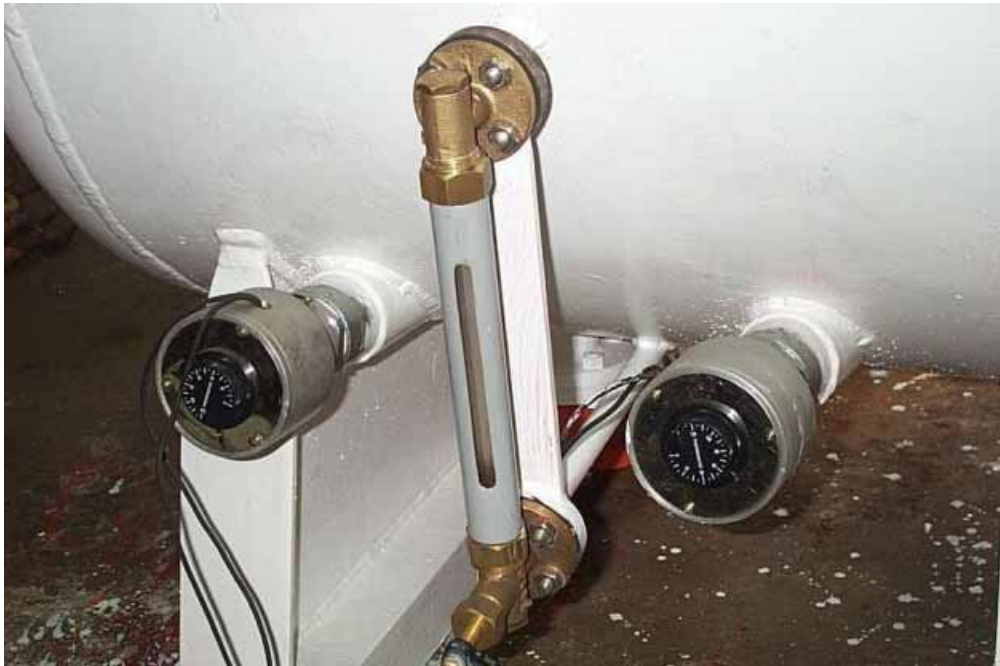
Photo. 2.3 Electric heater for heat supply unit
